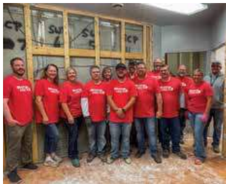
SVUW DAY OF CARING – Employees rolled up their sleeves to demolish the old Knowles Jewelry building. The work contributed to an area-wide Day of Caring through the Souris Valley United Way.
